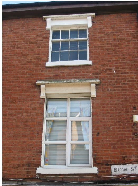
Fig. 4 Unsympathetic modern window replacement.
