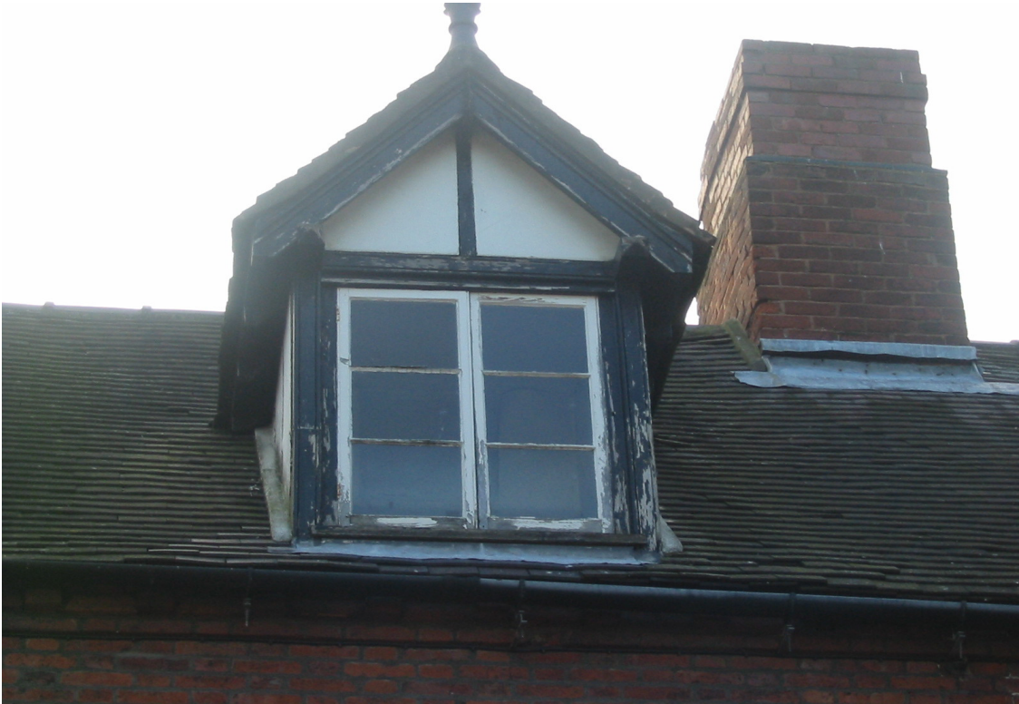
Fig. 1 Traditional detailing in need of repair.
