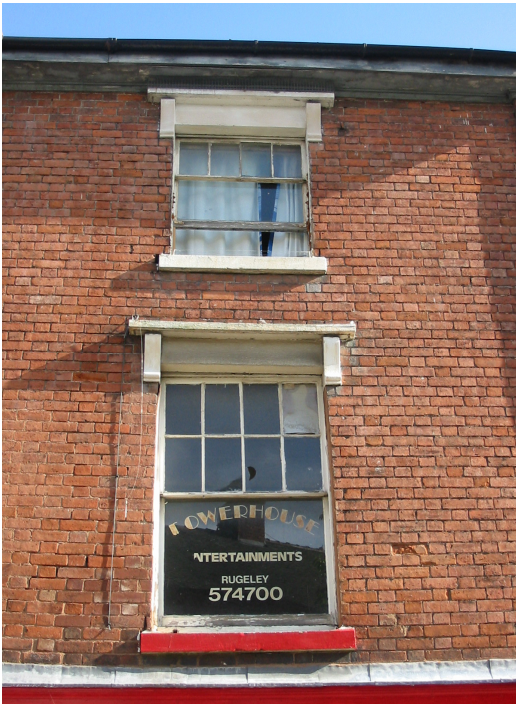
Fig. 3 Traditional windows in need of repair
