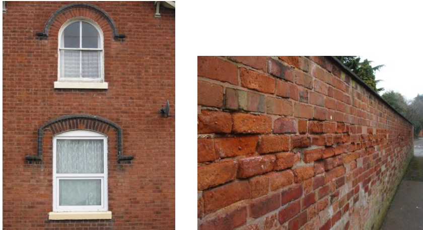
Fig. 14 Comparison of original and replacement UPVC windows; decay of a brick boundary wall
