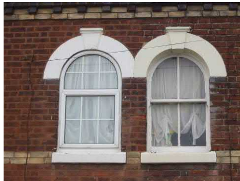
Fig. 12 comparison of original and replacement windows
