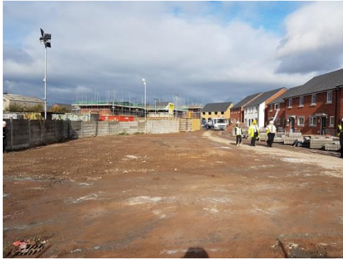
Figure 6 - the approach road to the rest of the housing estate. This will have the road and 4 parking bays
